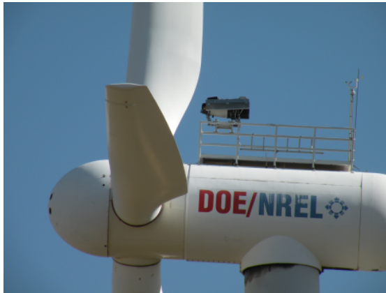
Figure 3.1: The SpinnerLidar with its mounting platform mounted on the nacelle of the research turbine CART3 at the National Renewable Energy Laboratory (NREL), Colorado, USA. Photo courtesy of Marijn Floris van Dooren.
