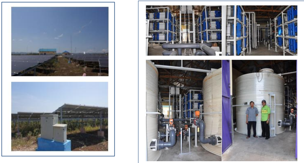
b) Examples of parts of installed power generation that belonged to Sumba smart microgrid project
